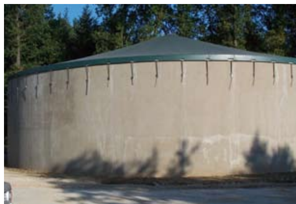
Photo 5: Covered digestate storage tank
