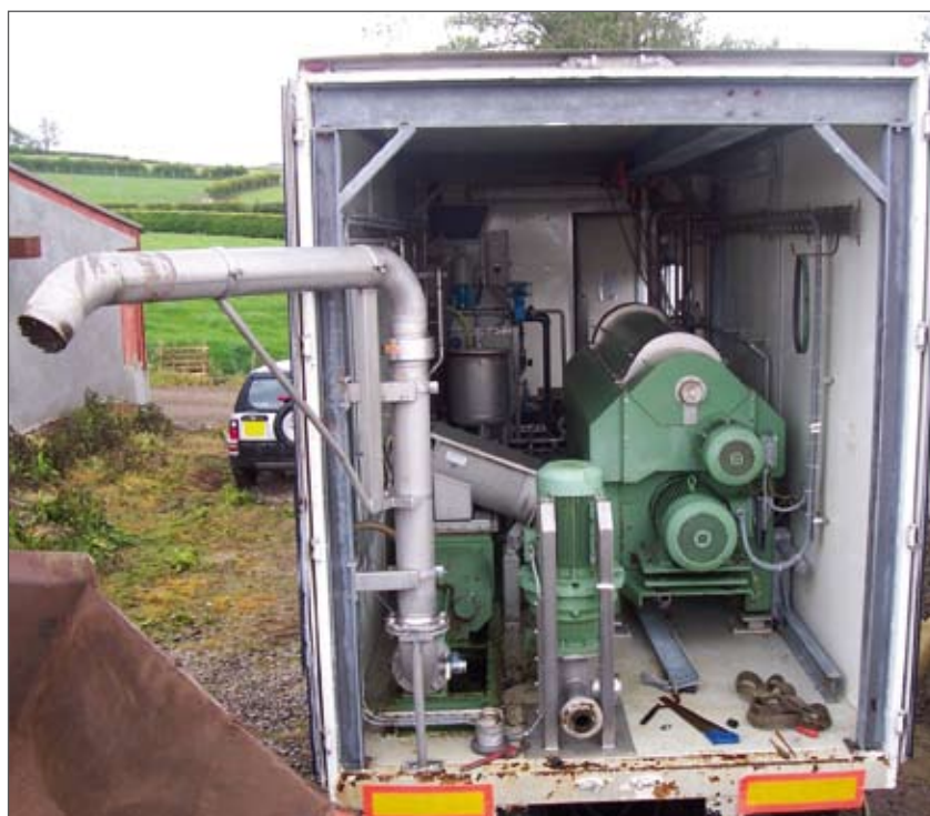
Photo 9: Decanter centrifuge mounted in a trailer unit for use in different locations
